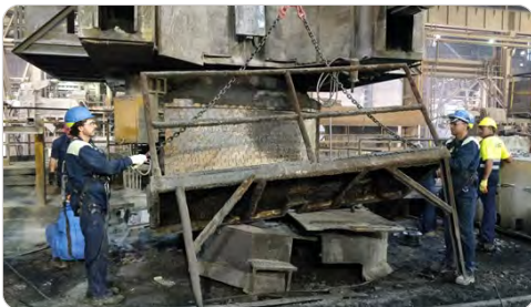
Picture 1: Old platform hooked. Picture courtesy of Acerinox Europa.
